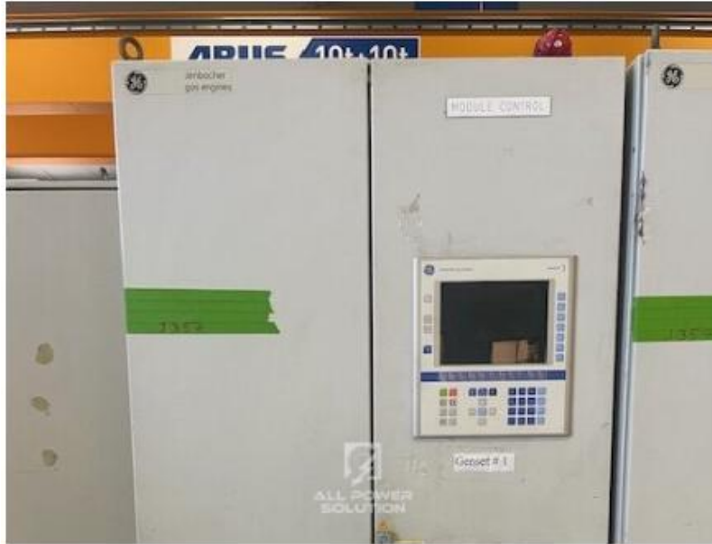
Figura 21. Panel de control Fuente (All Power Solution, 2023)
